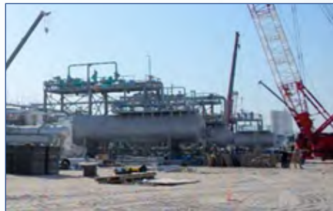
OIL TRAIN HP LP MP SEPARATION SKIDS
