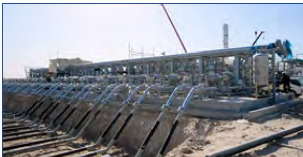
INLET MANIFOLD 50000 BOPD
