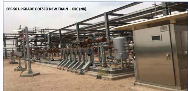
ESDV & AIR RECEIVER TANK
