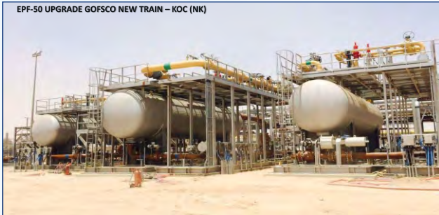
CRUDE SEPARATORS (HP MP & LP)
