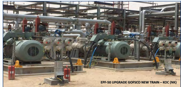
CRUDE EXPORT PUMPS
