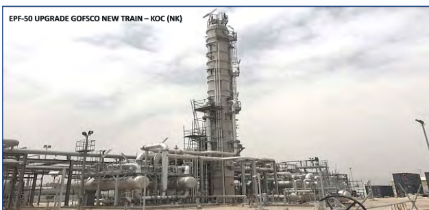
STABILIZER COLUMN, SIDE BOTTOM REBOILERS & WATER DECANTER
